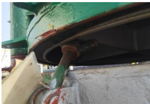
Figure 5. Condition of Rusty Manhole Threads
