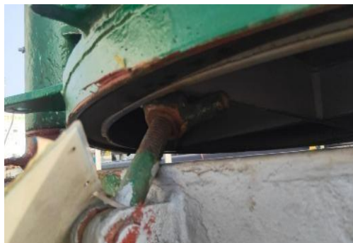
Figure 5. Condition of Rusty Manhole Threads
