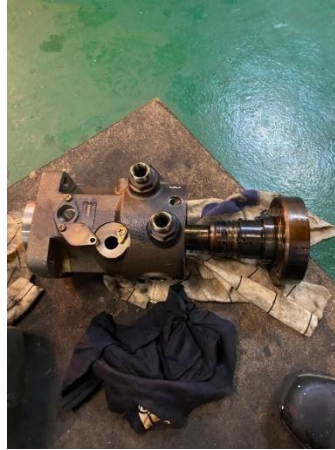
Figure 4. Fuel oil pump
