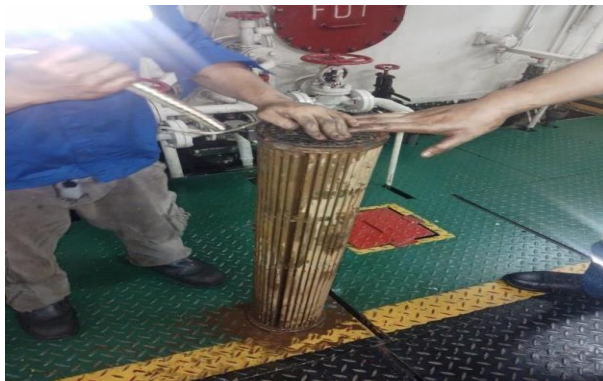
Figure 2. Leaking L.O Cooler Tube
