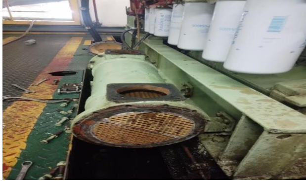
Figure 1. General View of the L.O Cooler on the Auxiliary Engine
