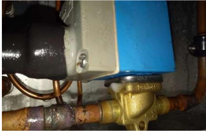
Figure 4. Leaks In Solenoid Valves And Pipes In Foodstuff Refrigeration Machine Systems
