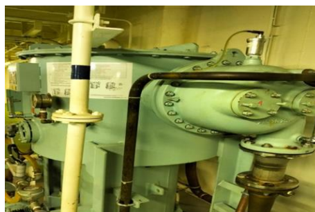
Gambar 3. Fresh Water Generator
