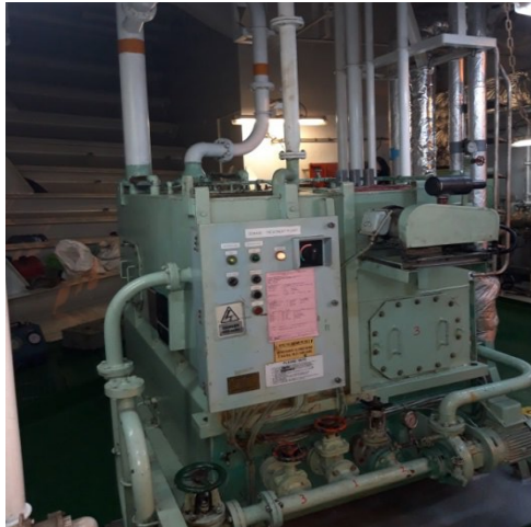
Figure 3. Sewage Treatment Plant MT.SWORDFISH
