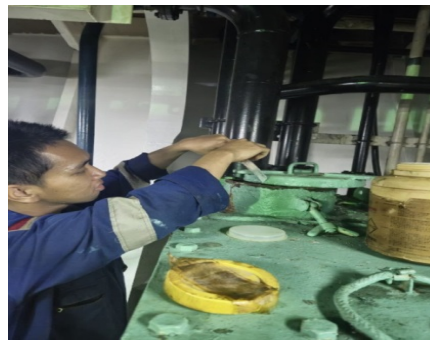
Figure 15. Oiler inserts Chlorine tablet
