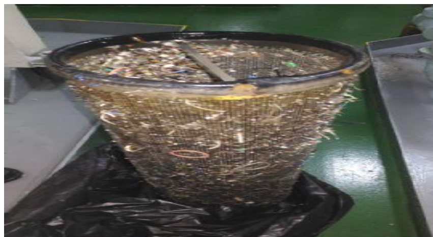
Gambar 4.2. Filter air laut Fresh Water Cooler
